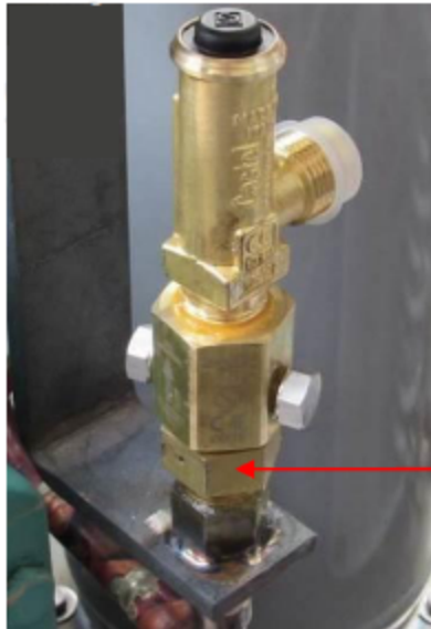
Rupture disc and safety valve
